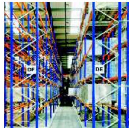
Narrow Aisle Pallet Racking
